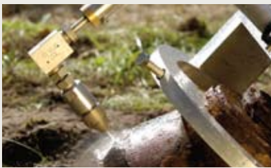
Cutting with Base Fuse Manipulator
